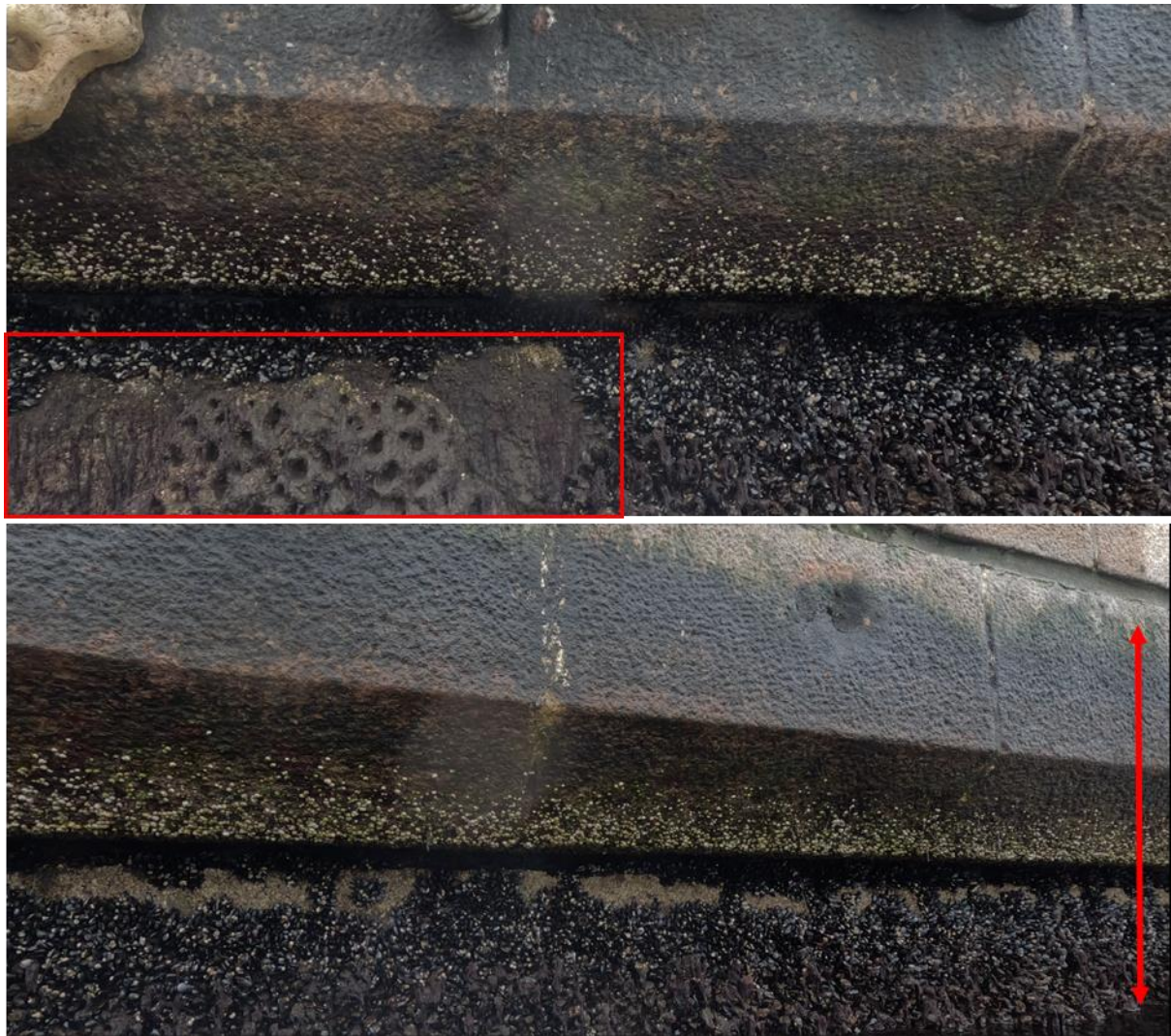
Figure 19. Living seawall (top) and living seawall control (bottom) above the waterline. The red rectangle outlines an example of a cleared area for reef panel installation. The difference between the water level during fieldwork and the usual waterline (approximately 0.5m) is indicated by the red arrow.
