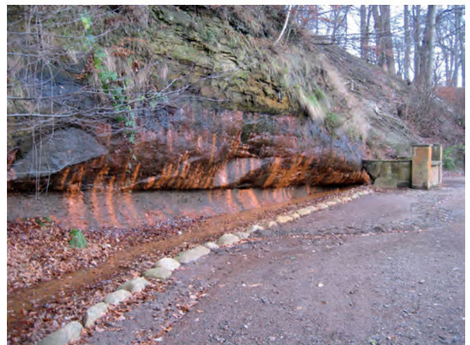
Ramlösa well. Water is still leaking out from a rock of sand stone.
